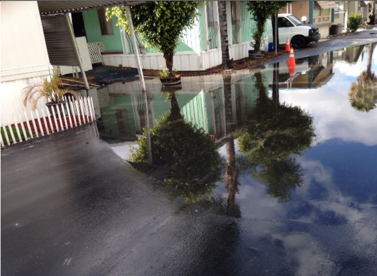
Above is a picture of the roadways that flood and water stands for a long period of time.
